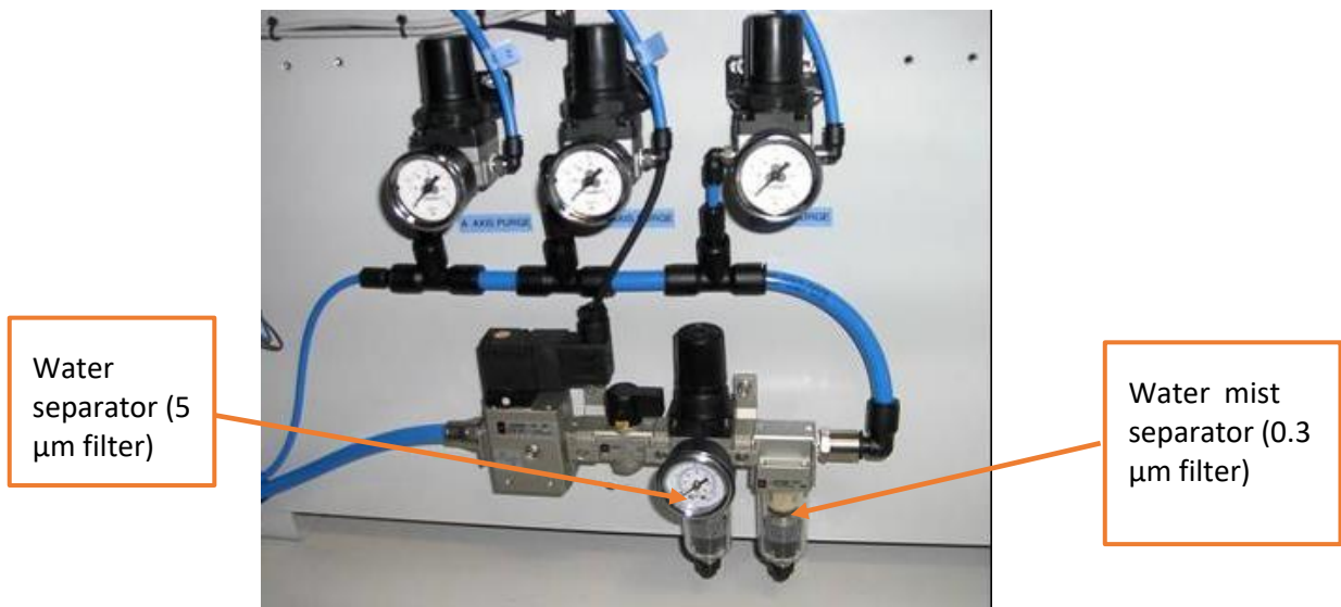
Figure 1 - Air service unit
